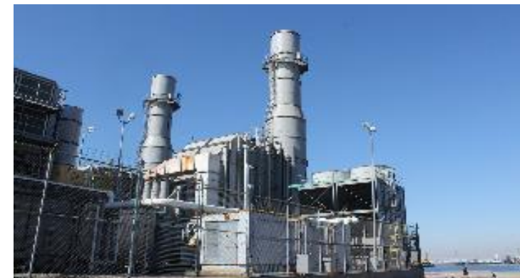
Captive Thermal + Waste Heat Plants (Total capacity of 161.5 MW)
